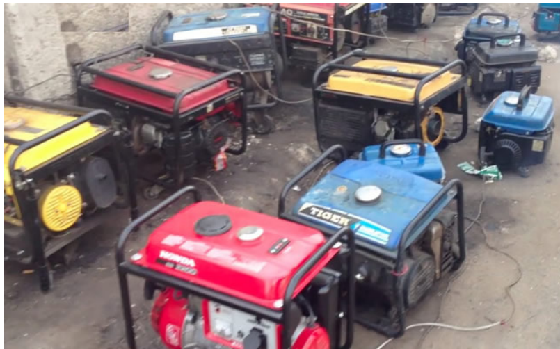
Difficult to maintain individual generators in microgrids
